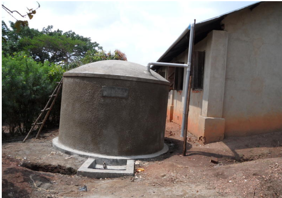
Complete constructed water tank on at Kashongi 1 primary school in kashongi sub county Kiruhura district(MMHF photos)
